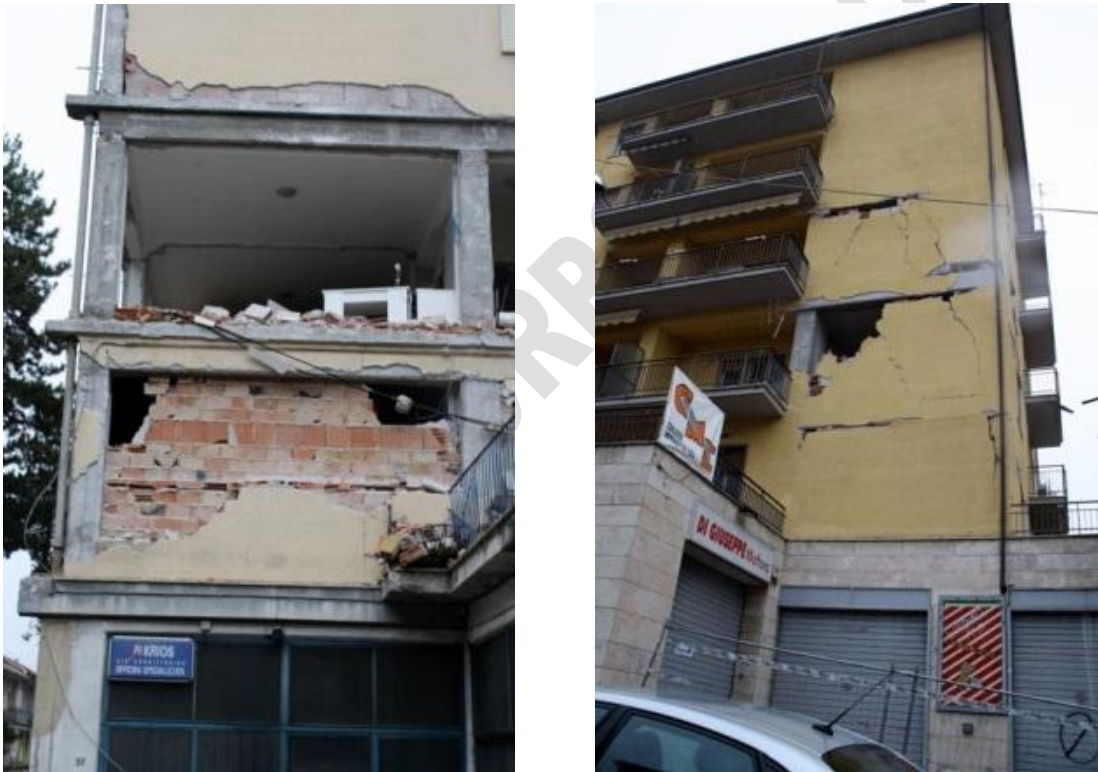
Figure C7.7: Masonry infill frame damage observed following the 2009 L'Aquila earthquakes (Win Clarke)
