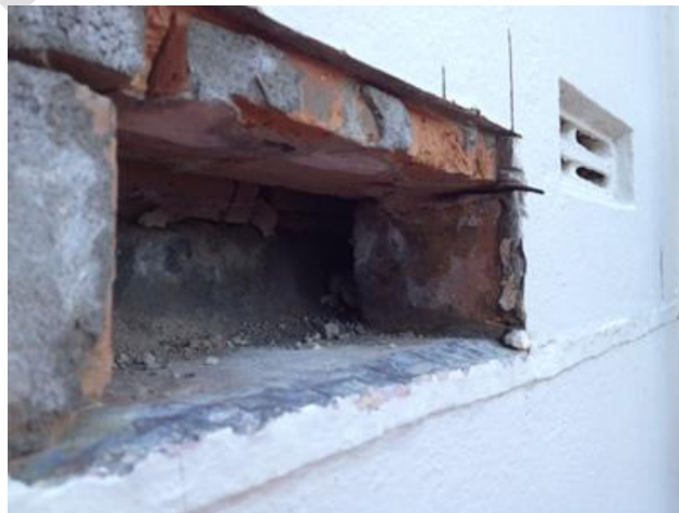
Figure C7.2: Typical clay brick cavity infill wall construction with plaster façade and single brick removed, exposing the air cavity separating two single wythes of clay brick (Kevin Walsh)
