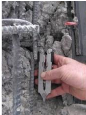
Figure 3 Fractured bars in lightly reinforced wall
