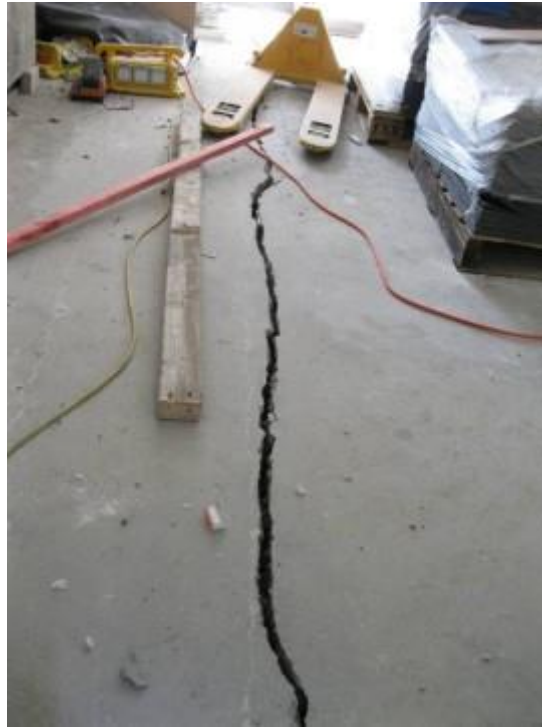
Figure 4 Tearing of insitu topping of precast flooring caused by frame elongation
