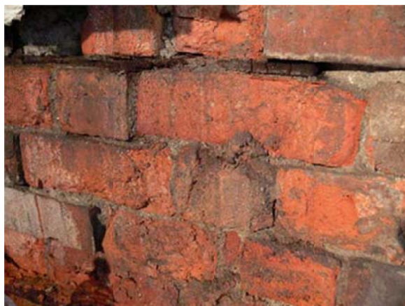
Figure 10.52: Severely degraded bricks and mortar due to moisture ingress (Ingham & Griffith, 2011)
