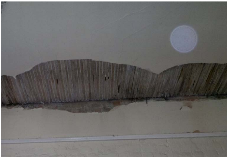
Figure 10.32: Lath and plaster ceiling. Note that stresses where shears are transmitted to the wall have caused the plaster to delaminate from the timber lath.
