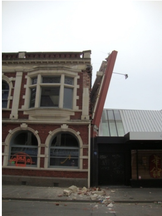
Figure 10.39: Out-of-plane instability of wall under face load due to a lack of ties between the face-loaded wall and rest of the structure (Richard Sharpe)
