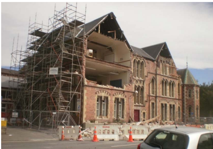
Figure 10.14: A lack of connection of the walls parallel to joist and rafters with diaphragms and return walls leading to collapse of wall under face load
