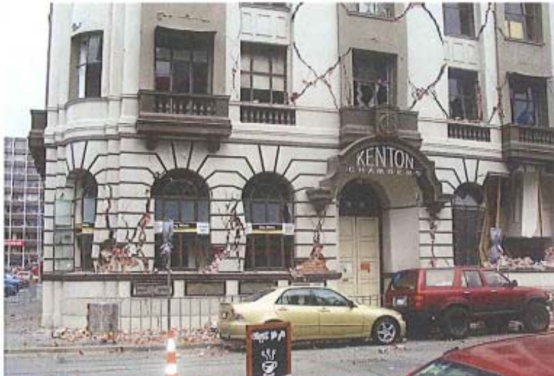
(a) Diagonal tension cracks to a brick pier. Note splitting of bricks (Dizhur)
