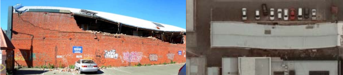
Figure 10.31: Out-of-plane wall failure due to excessive roof diaphragm movement (Dizhur et al, 2011)
