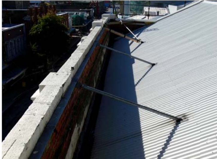
Figure 10.27: Parapet bracing. Note a lack of vertical tie-up of the parapet (Dmytro Dizhur)
