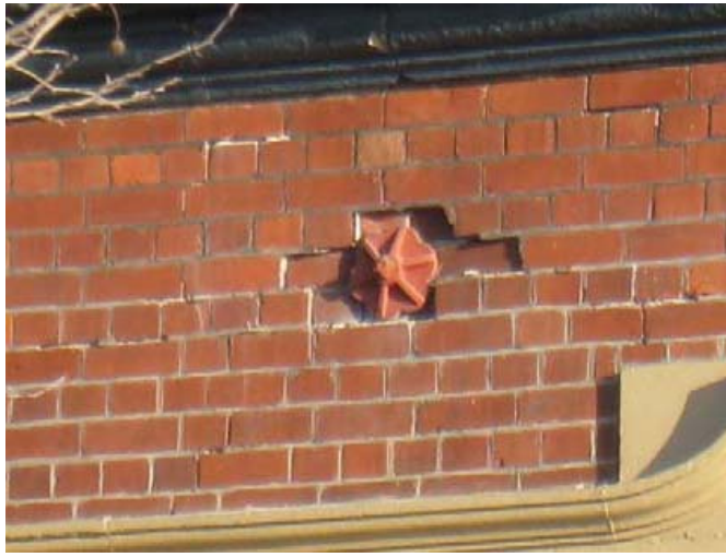
Figure 10.34: Plate anchor on verge of punching shear failure (Dizhur et al, 2011)
