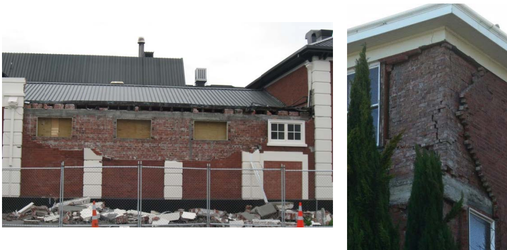
Figure 10.41: Failure of URM cavity walls (Dizhur)
