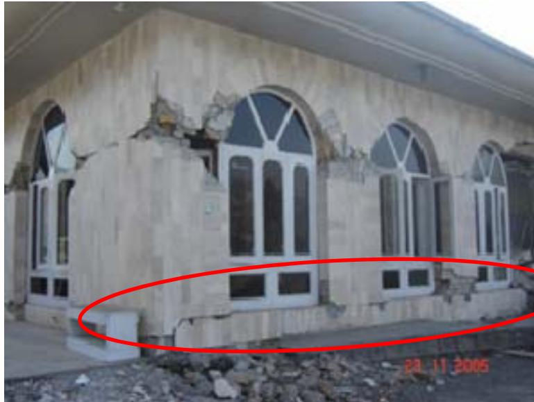
Figure 10.43: Rocking and delamination of bricks of a one-storey unreinforced brick masonry building with reinforced concrete roof slab (Bothara & Hiçyılmaz, 2008)
