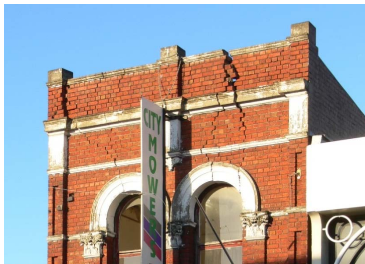
Figure 10.21: The wide cracks through bond beams indicate a lack of reinforcement in the beam (Dizhur)
