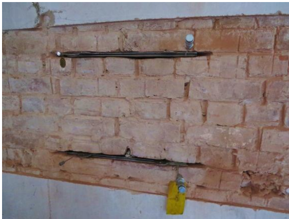
(a) Cutting mortar bed-joints and insertion of flat jacks into clay brick masonry
