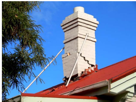
(b) Chimney at onset of falling ( Dizhur)
