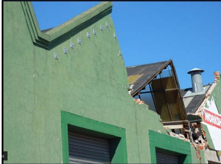
Figure 10.40: Collapse of gable wall. Note a secured gable end that survived earthquake loading and a companion failed gable end that was not secured (Ingham & Griffith, 2011)
