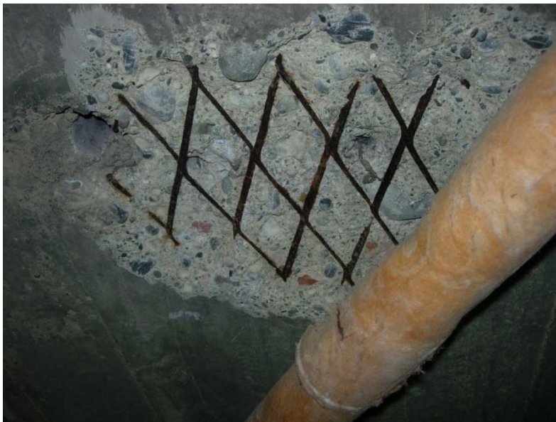
Figure 10.11: Concrete slab with expanded metal lath reinforcement. Corrosion of the lath from carbonation of the concrete over time has caused the concrete to spall.
