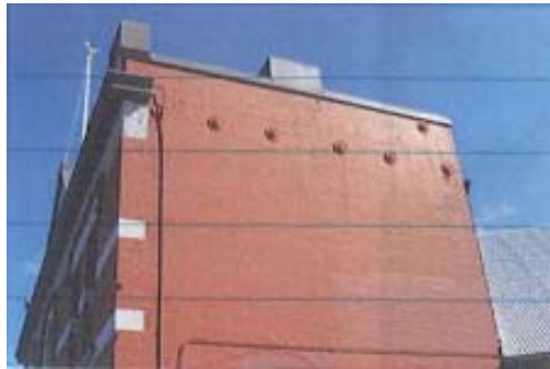
(a) Post-September 2010 event – minor visible damage
