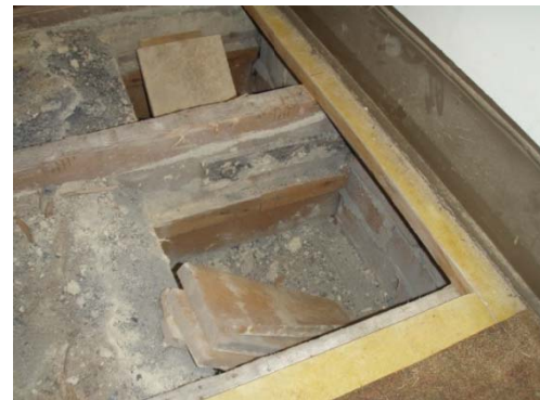
(b) Floor joist to wall connection. Note presence of steel strap (Matt Williams)
