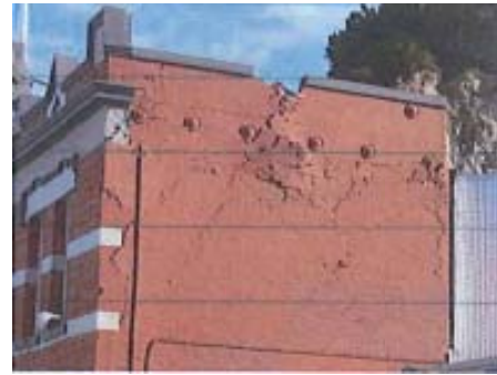
(b) Post-February 2011 event – wall section on verge of failure
