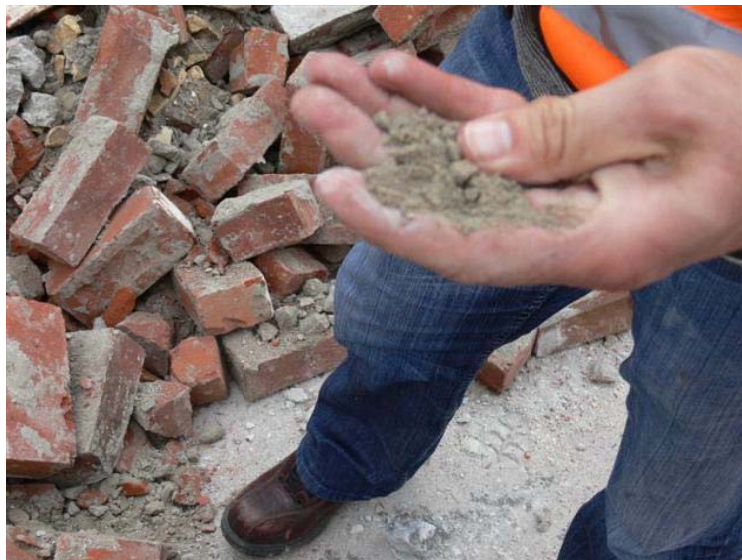
Figure 10.10: Soft mortar. Note the delaminated mortar from bricks in the background (Ingham and Griffith, 2011)
