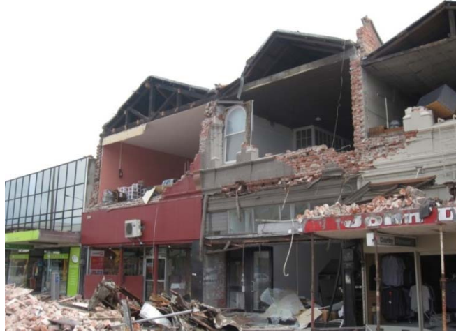
Figure 10.48: Face-load failure of URM façade exacerbated by outward loadings from downward force on canopy. Note the adjacent propped canopy did not collapse. (Dunning Thornton)
