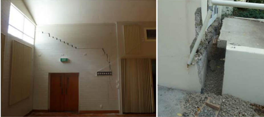
(a) Large diagonal cracks and lateral movement of the access ramp caused by ground movement
