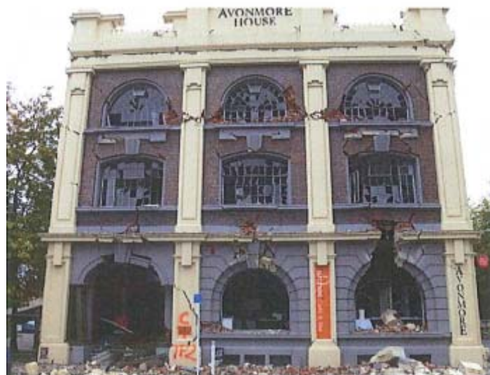
Figure 10.46: Failure of spandrels. Also note rocking of upper piers and corner cracking of the parapet (Dmytro Dizhur)
