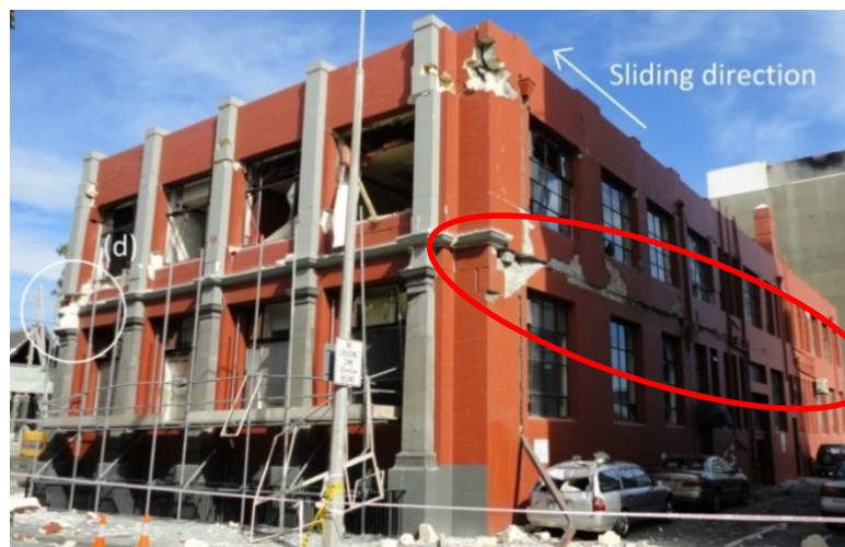
(a) Sliding shear failure along a defined plane at first floor level (Dunning Thornton)
