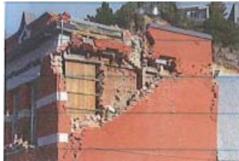
(c) Post-June 2011 event – wall collapse
