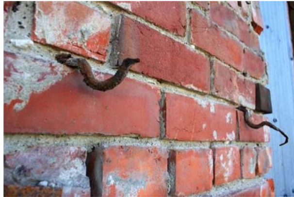
Figure 10.53: Metal cavity ties in rusted condition (Dizhur et al, 2011)
