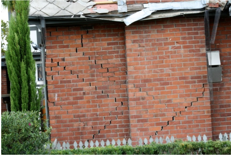
(b) Stair-step crack sliding, in walls with low axial loads (Bothara)
