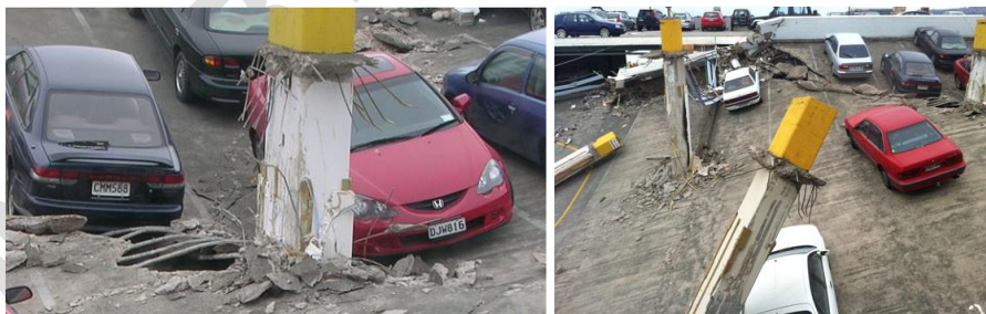
Figure C2G.2: Collapse of flat-slab system observed in Christchurch (from Kam et al., 2011)
